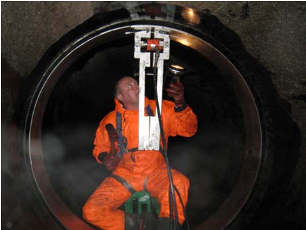
Setting the sleeve against the pipe wall by using a rubber hammer
